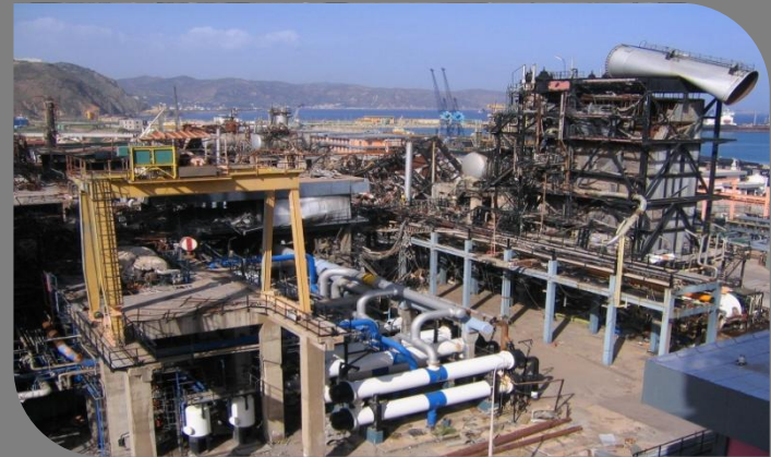
Skikda LNG plant, Algeria (2004) LME induced explosion in cold box 27 killed, 72 injured, cost US$30,000,000
